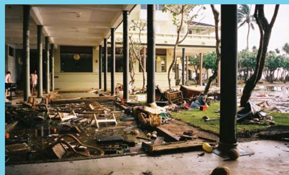
Debris in the swimming pool and lobby as a result of the tsunami waves.
